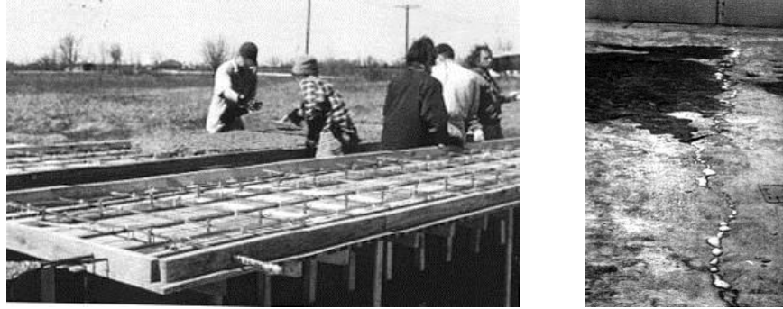
Figure 6) Left, photo of fabrication of bridge decks. Right, photo of released repair adhesive [6].
