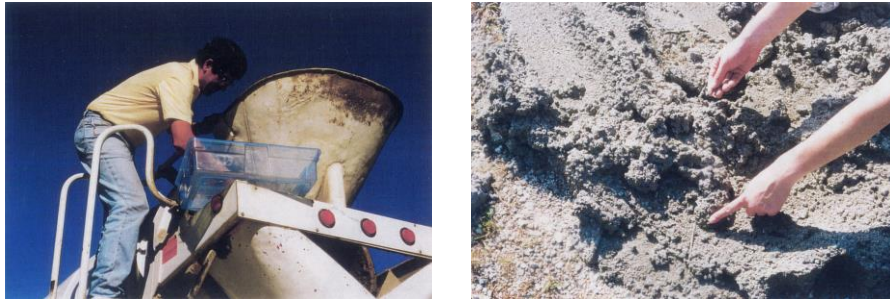
Figure 5) Fibers being thrown into the cement mixer at the site, on the left, and they survive after mixing in the bridge concrete, on the right.
